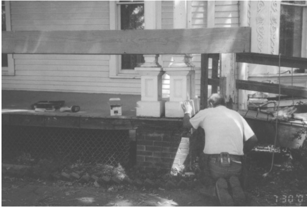
Vernon Smith from V. H. Builders raises corner of front porch to replace sill that had deteriorated under the front edge
