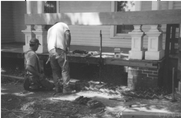
Vernon Smith & Lyn Boston install new beam under front edge of the front porch
