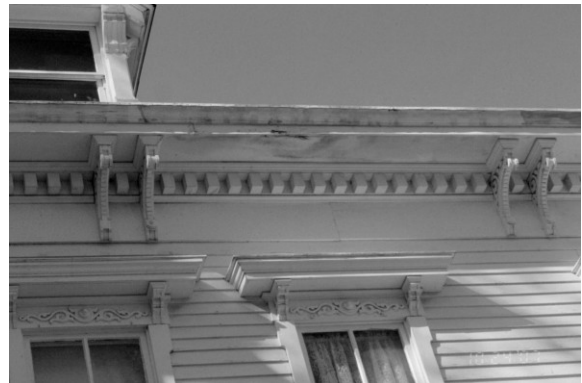
Museum needing repair & paint
